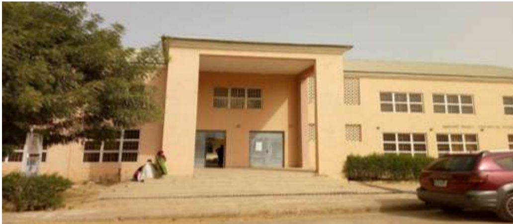
Plate II The façade of the School of Post graduate Studies, ADUST Wudil. Showing no element of vertical or horizontal shading device.
