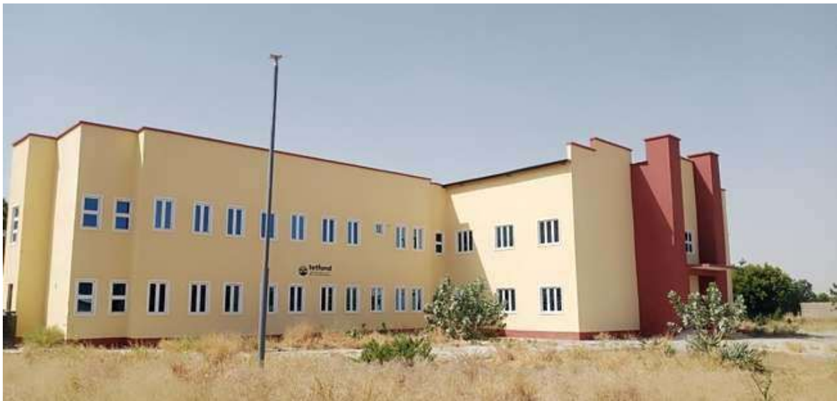
Plate 3: New School of Environmental Studies Complex – 2019 Special Impact exhibiting wrong orientation and lack of effective shading devices on the wall facades
