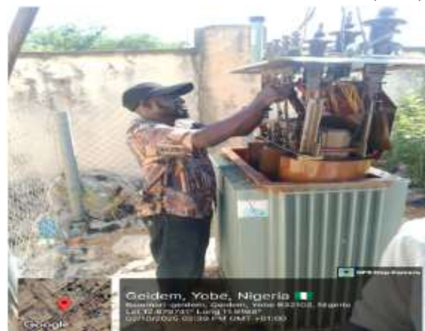
Figure 4: Detecting fault for proper repair in 33KVA power transformer
